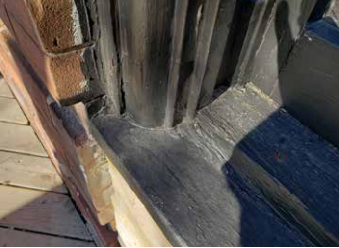
Figure 31: Typical condition of wood windows, EVOQ
