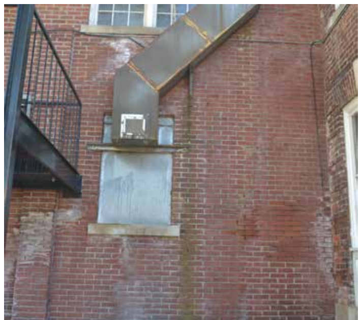
Figure 30: Typical conditions of masonry on the west elevation, EVOQ
