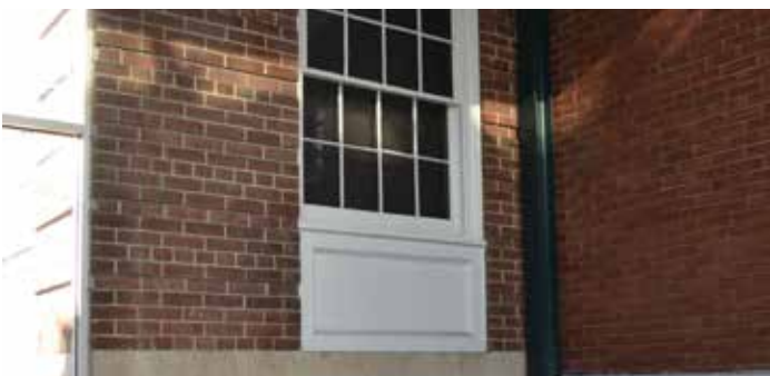
Figure 29: Typical conditions of masonry within the enclosed vestibule, EVOQ
